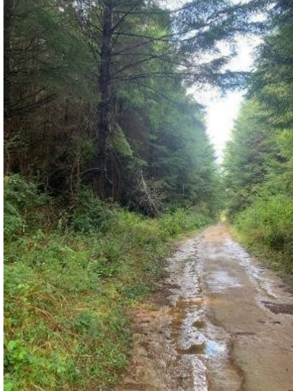
Figure 2. Road Erosion near Widow White Creek on Main Road
