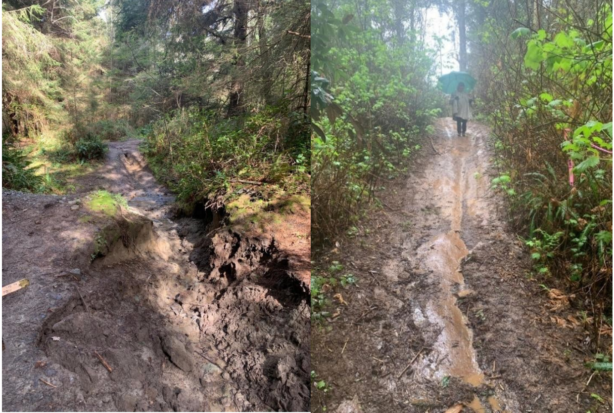
Road point 1.3 South side of Widow White Creek roadGPS 40.56968 -124.4847. Road Reconstruction site road approach needs to be disconnected from the Watercourse.
