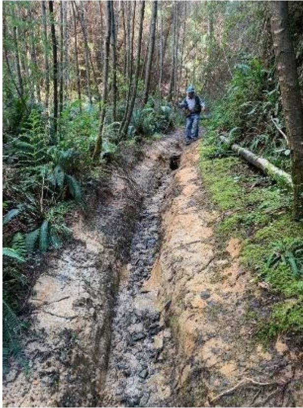
Figure 1. Road Point 1.9 Former truck road requiring reconstruction
